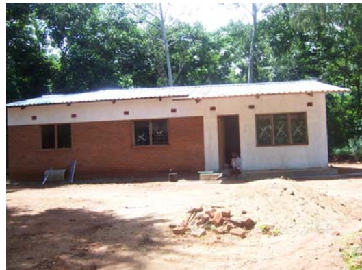
Below is a senior staff house which is on the finishing stage also funded by Cordaid
